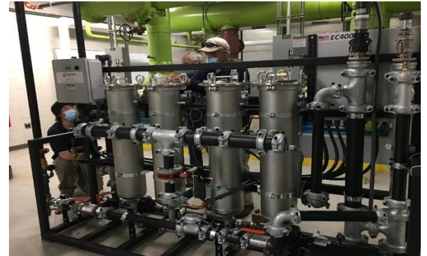
Installation on a 3,000 ton capacity central chilled water plant.
