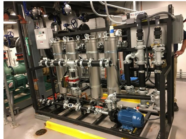
Installed EC-4000 ElectroCell skid
