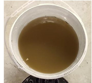
Debris removed from condenser water after 1 week of operation
